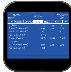
UPS Cabinet Control Panel
